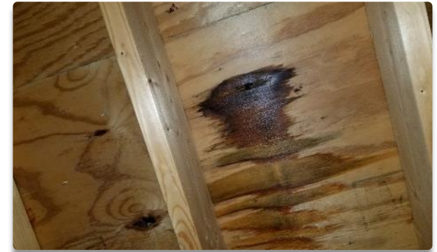
Water damage on ceiling
