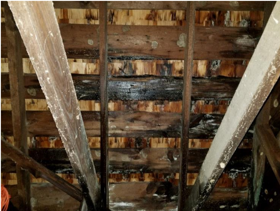
Water damage in the smoke house.
