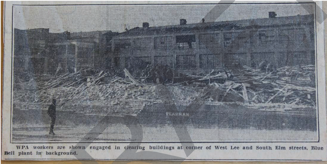
Figure 4. Tornado Damage at the Blue Bell Company Plant, April 7, 1936. Greensboro Daily Record , 4.
