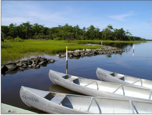
A Living Shoreline constructed at Pine Knoll Shores Aquarium, North Carolina. Photo from North Carolina Coastal Federation.
