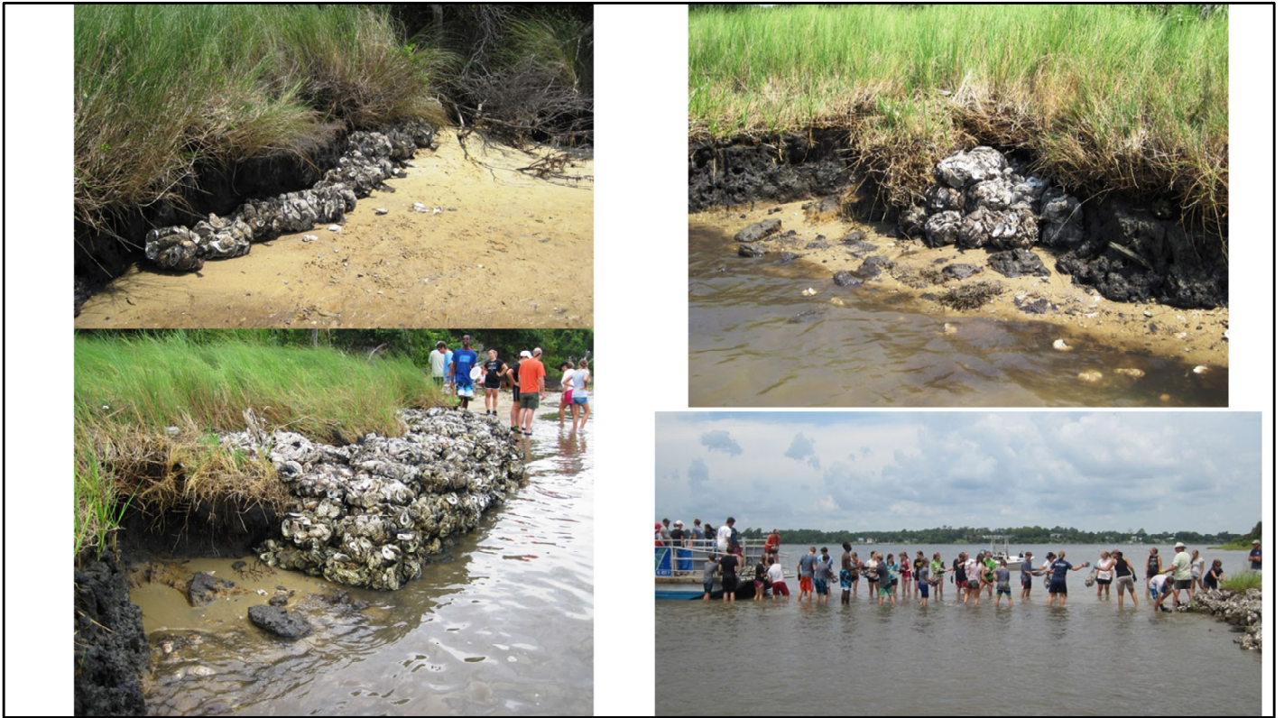
This marsh toe revetment, constructed from bags of loose oyster shell, was built by volunteers.
