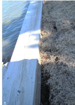
Scour landward of the wall
