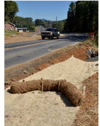
Design: Erosion and Sediment Control Devices on NC 88 in Jefferson, NC
