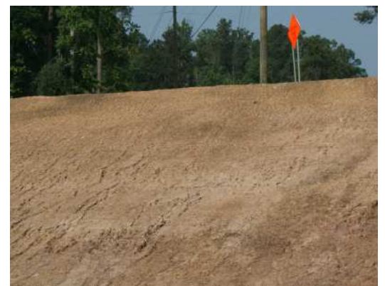
Rill Erosion: The Department is looking at other alternatives to stabilizing erodible slopes other than temporary mulch.
