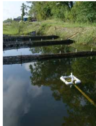
Design: Erosion and Sediment Control Devices on NC 17
