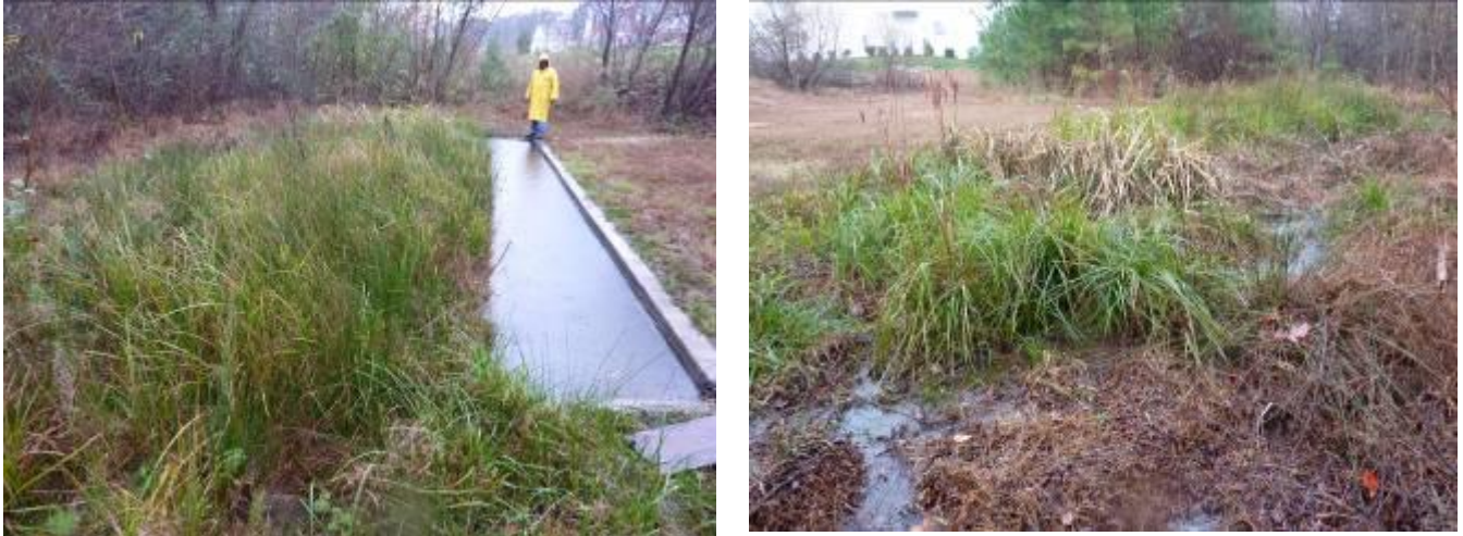
Figure 13: Unmaintained Blind Swale and Unmown FS
