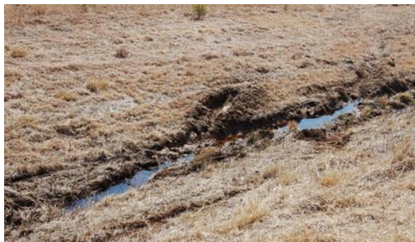
Figure 6: Rutting Due to Mowing
