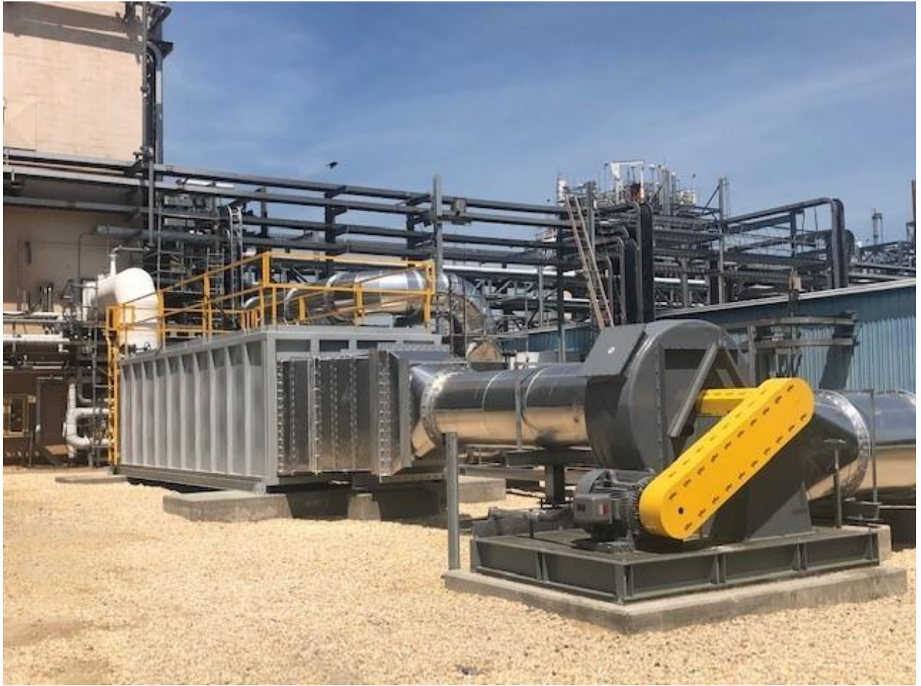
Vinyl Ethers South Carbon Adsorber Unit Installed in June 2019
