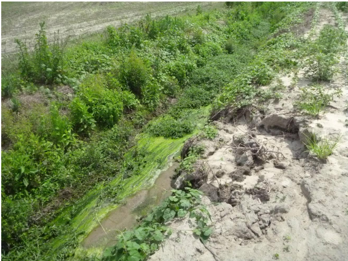
Figure 9. Bank failure along a ditch with no vegetated buffer at a stream assessment site (SA008) in the Sevenmile Swamp subwatershed (SMS 04).
