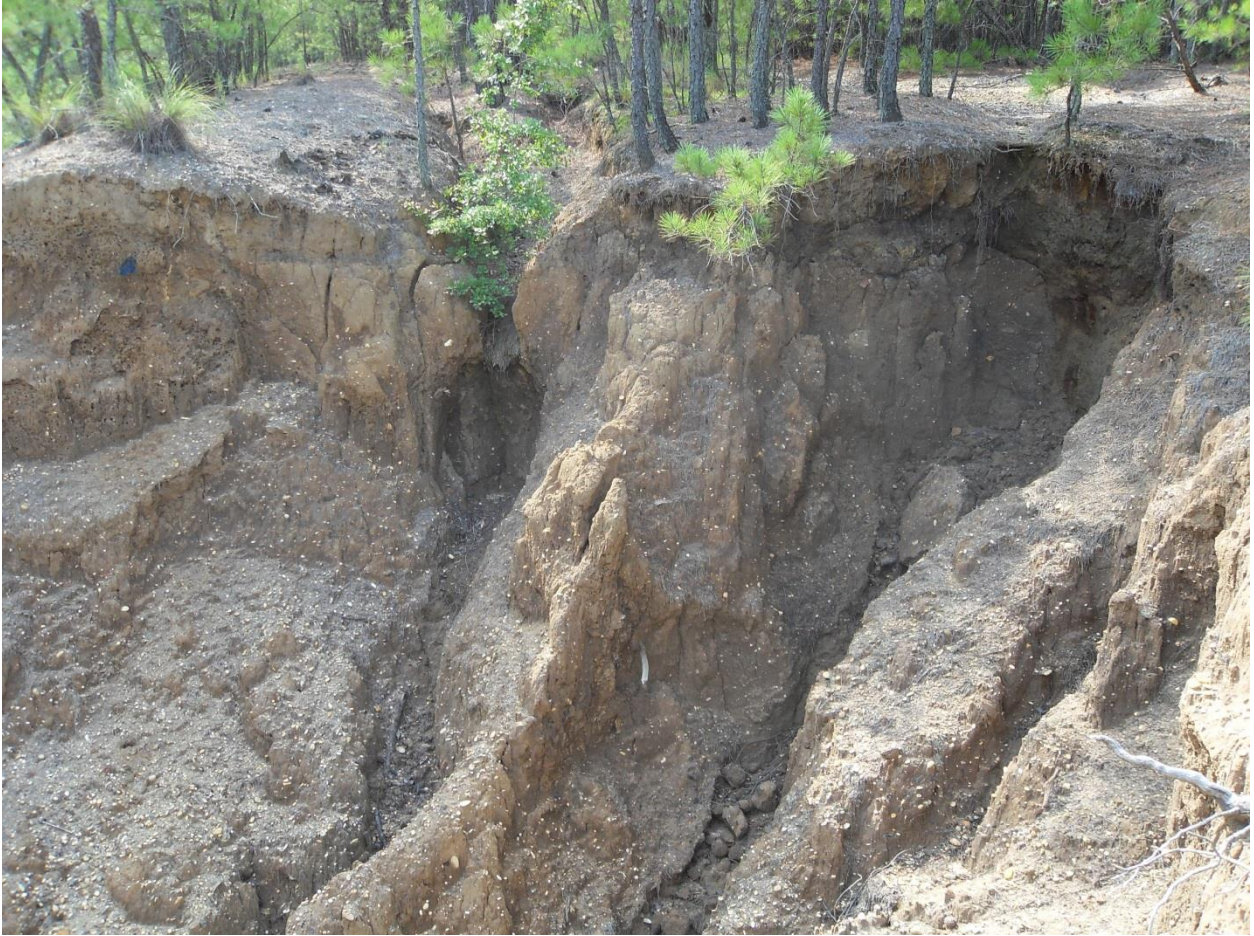
Figure 13. WRO-064 with severe erosion of unconsolidated materials. This site is in BDS 01.
