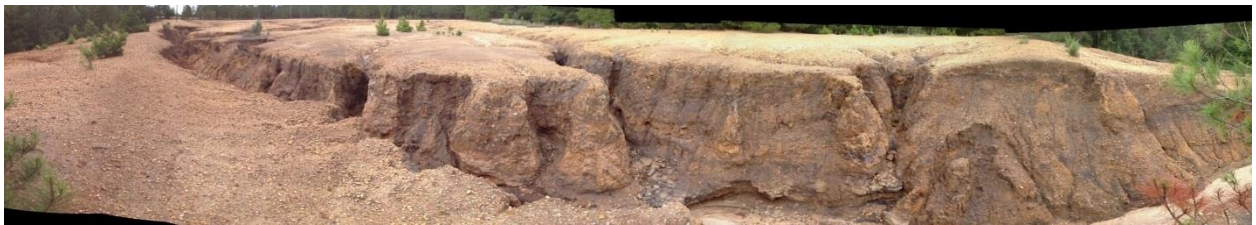
Figure 10. WRO-063 panoramic image showing massive erosion and headcuts. This site is near Beaverdam Swamp in BDS 01.
