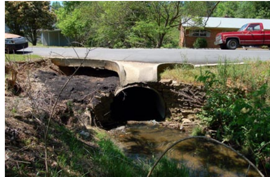
Figure 2: Failing Stormwater Culvert in Little Alamance Watershed
