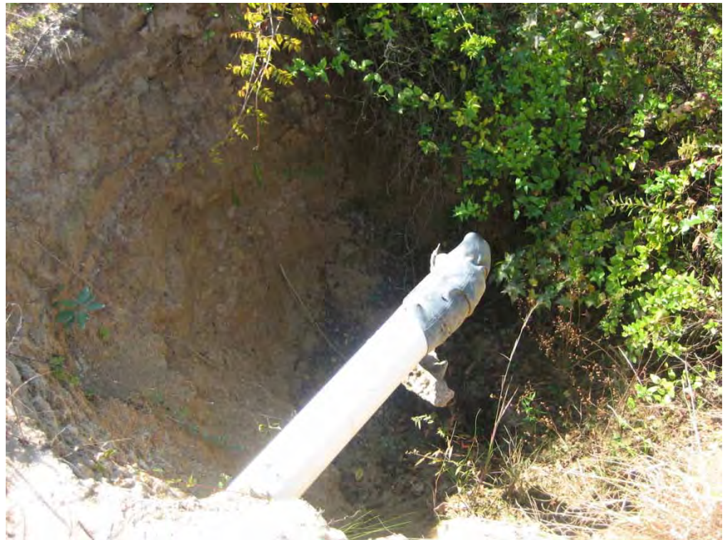
Repairing the pond outfall pipe and pond dike provides stormwater retrofit opportunity
