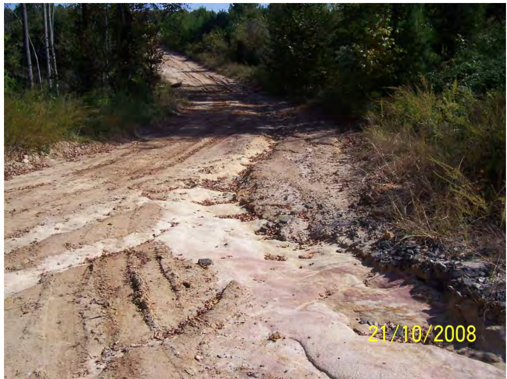
Evidence of erosion resulting from exposed soil
