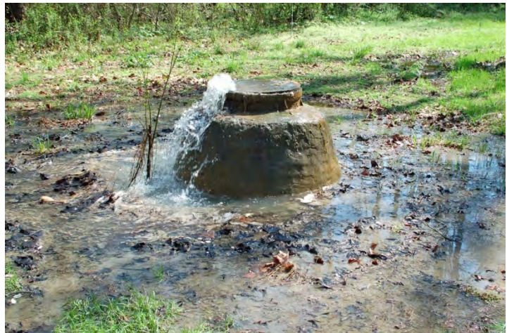
Figure 40: Sewer Overflow in Eden
