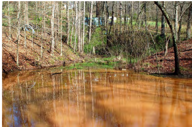
Figure 27: Failing Farm Pond & Spillway, Matrimony Creek, PTRC 2012
