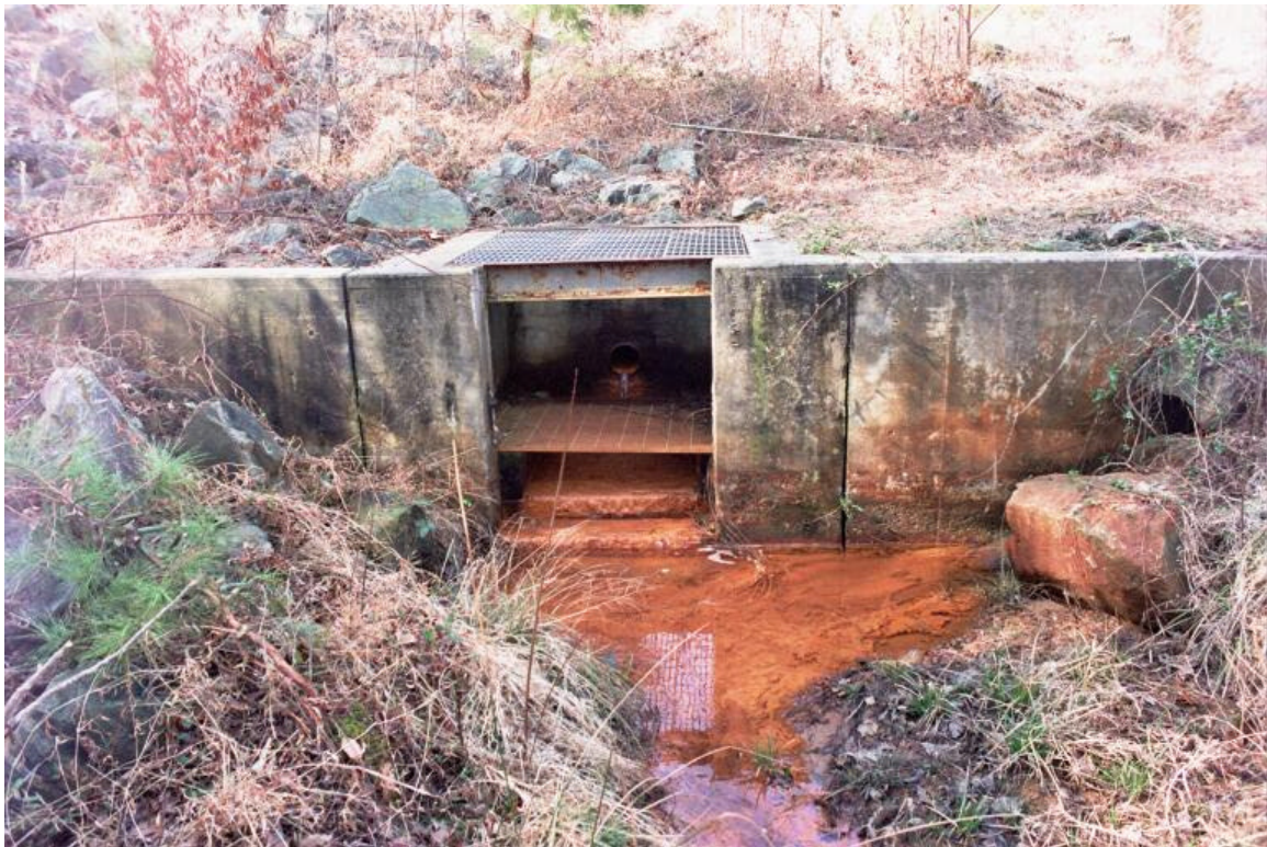
30. Ash Pond Dam. East weir. Minor sediment accumulation in outlet channel.
