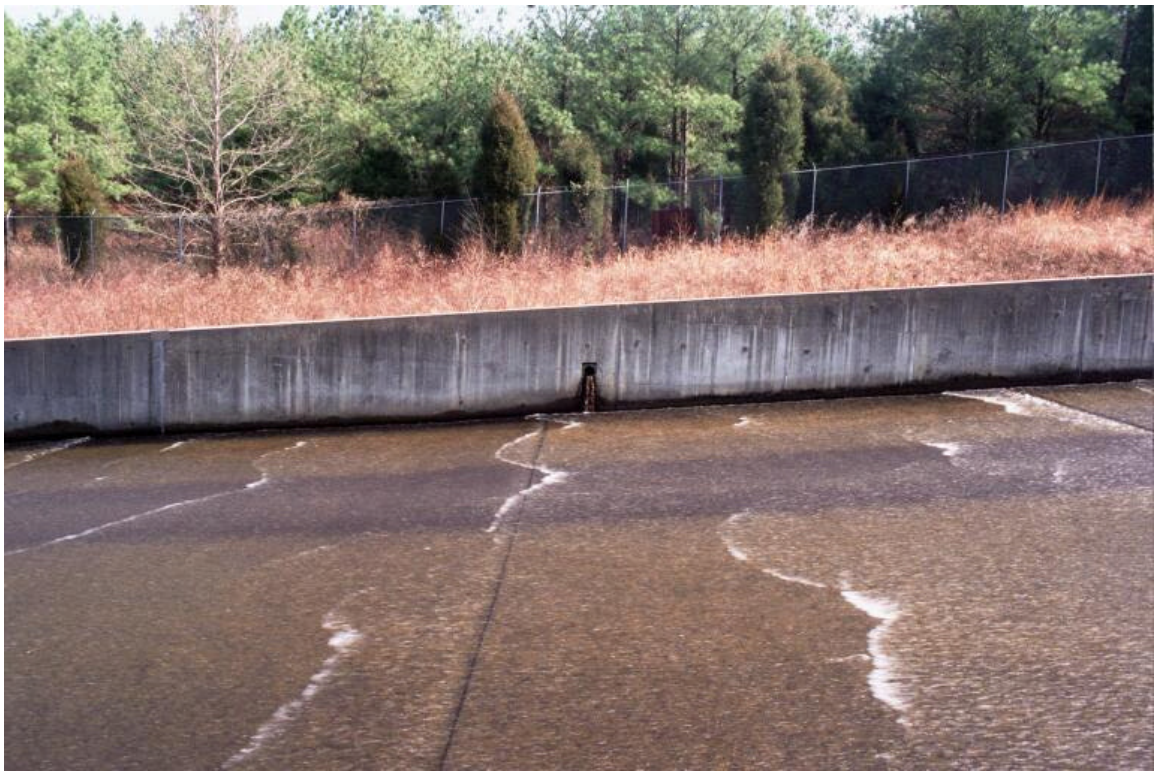
16. Mayo Creek Dam. East side wall of primary spillway showing active weep hole.
