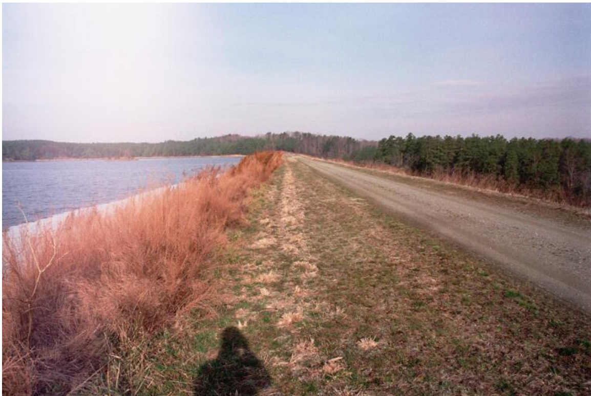
22. Ash Pond Dam. Crest and upstream slope. Vegetation on slope is dead (sprayed).
