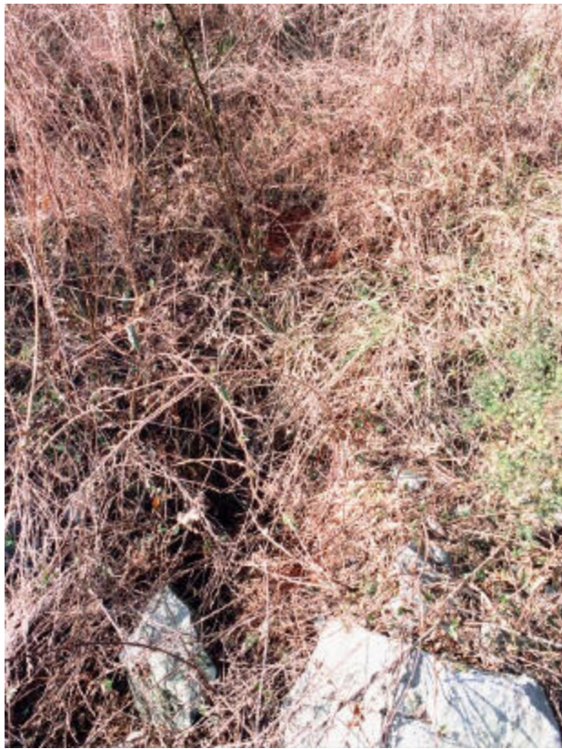
27. Ash Pond Dam. Hole at top of rock toe on west section.
