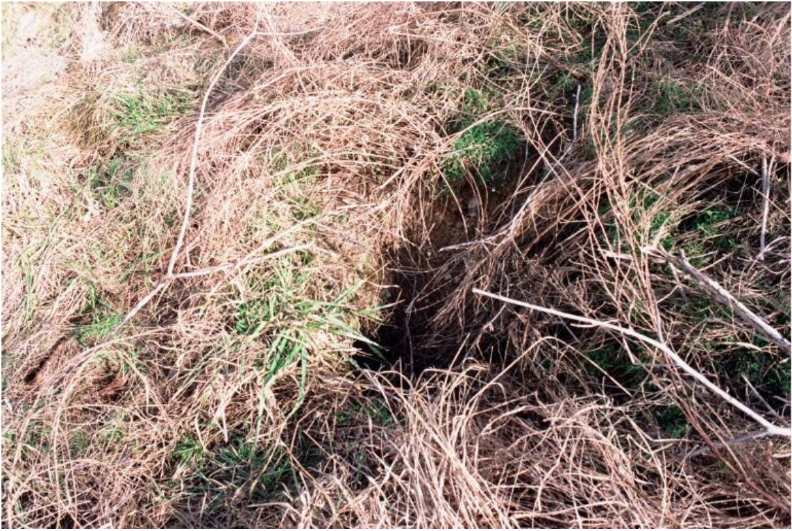
9. Mayo Creek Dam. Hole at top of rock toe.
