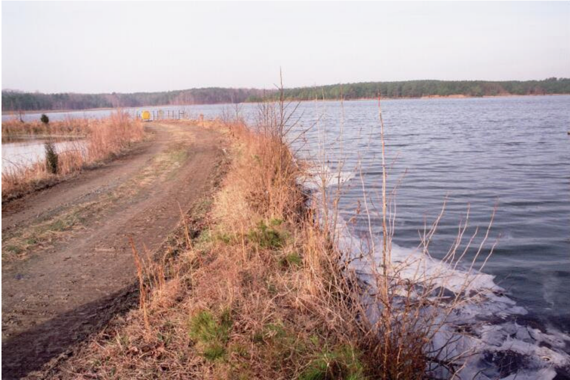
35. Ash Pond Dam. Upstream slope of secondary pond dike. Small trees need control.
