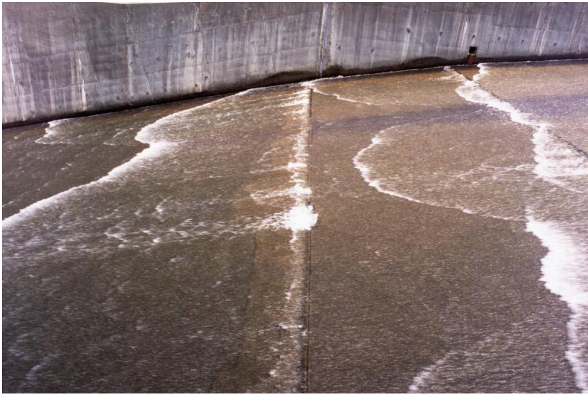
19. Mayo Creek Dam. Flow across joint 19. Disruption of flow at spalled concrete areas seen previously.
