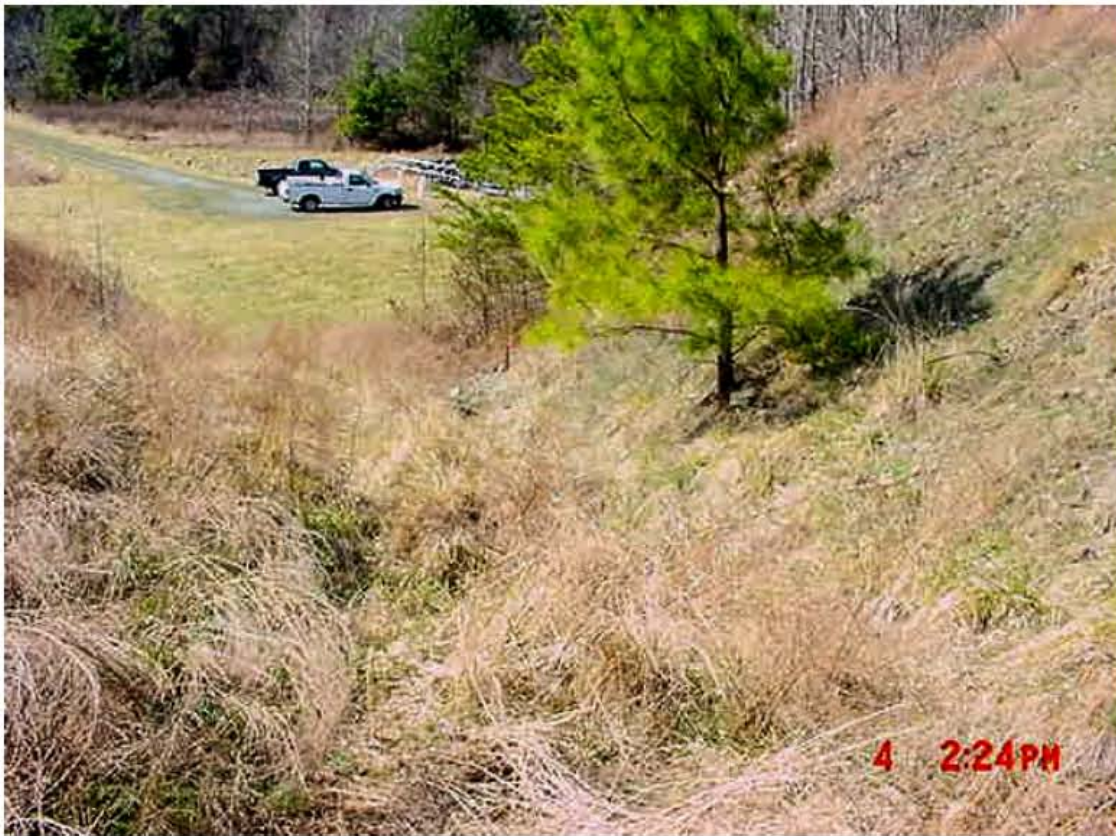
13. Mayo Creek Dam. East abutment-dam toe junction where slight seepage flow noted.
