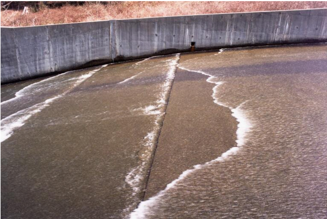
18. Mayo Creek Dam. Flow across joint 18. Slight disruption near center of spillway.
