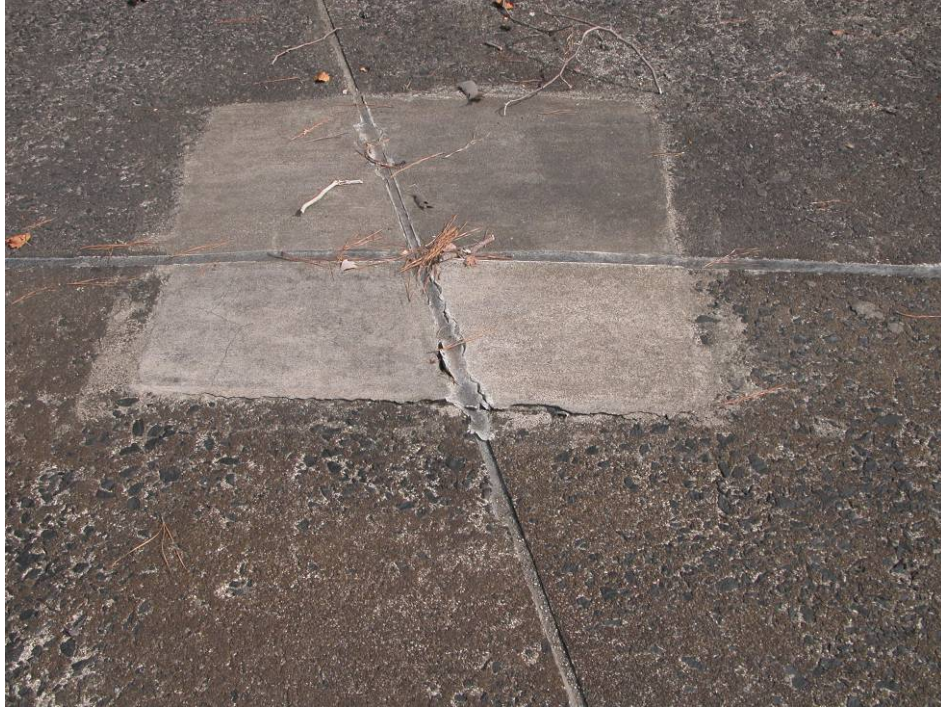
23. Main Dam – Patch with loose caulk on C12, D12, tight C13, D13 at junction C12, C13, D12, D13 (August 5, 2008).
