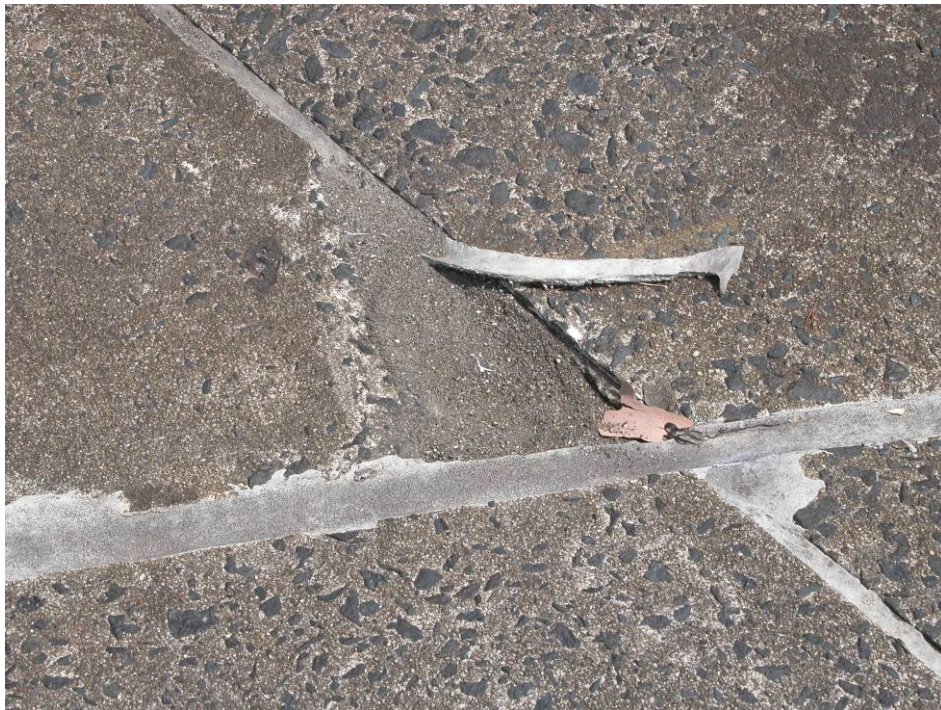
22. Main Dam – Patch eroded out and caulk pulled up (I11/J11 - August 5, 2008).
