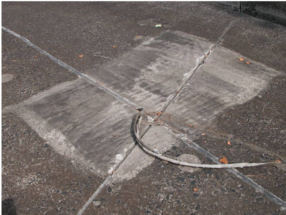
20. Main Dam – Patch at joint D12/D13 to joint D13 torn out; E11/E12 caulk torn out at D13 joint (August 5, 2008).
