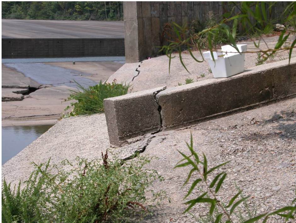
18. Main Dam – Old crack in concrete slope paving behind downstream end of spillway left retaining wall (August 5, 2008).
