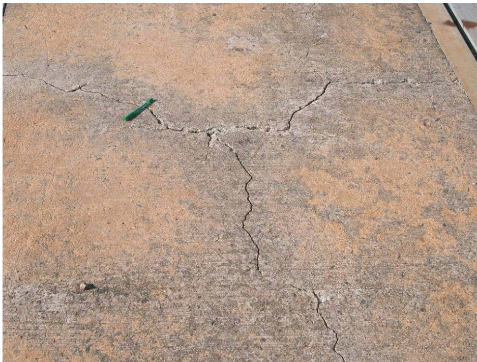
62. Afterbay Dam – View of cracking at crest of Pier 2.
