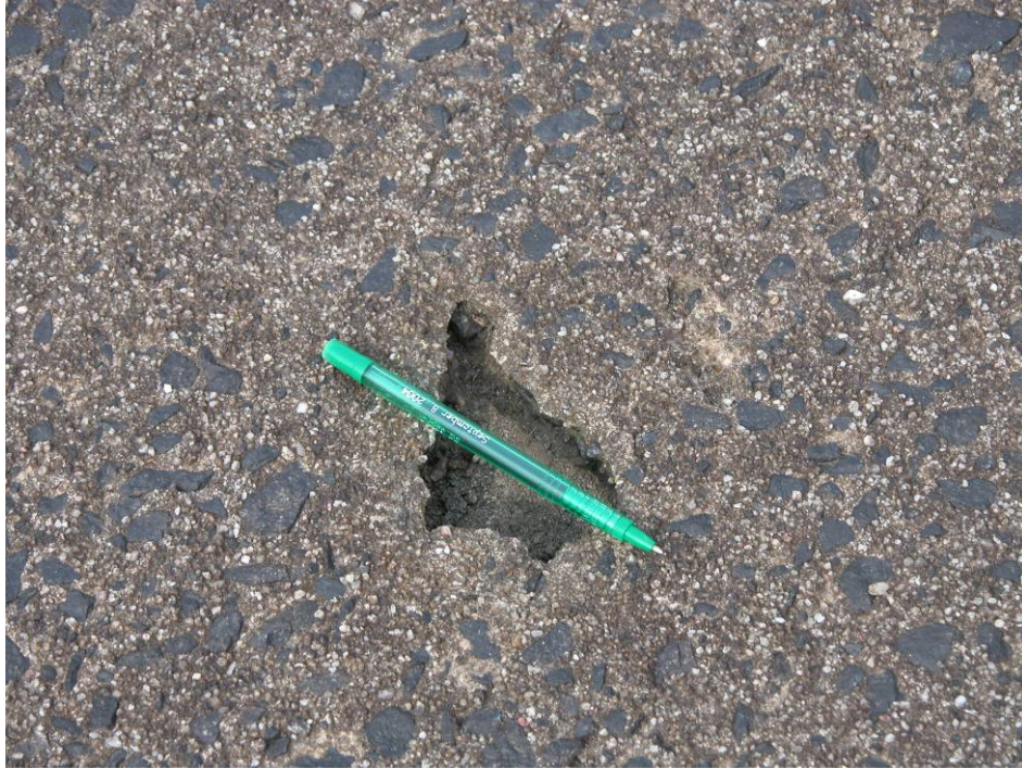
25. Main Dam – Aggregate popout hole 2 inches by 3 inches and 1.5 inches deep in section B5 (August 5, 2008).
