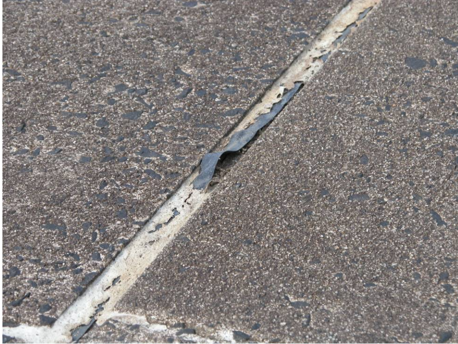
19. Main Dam – Example of tape over caulked joint pulled off (joint B11/B12 - August 5, 2008).
