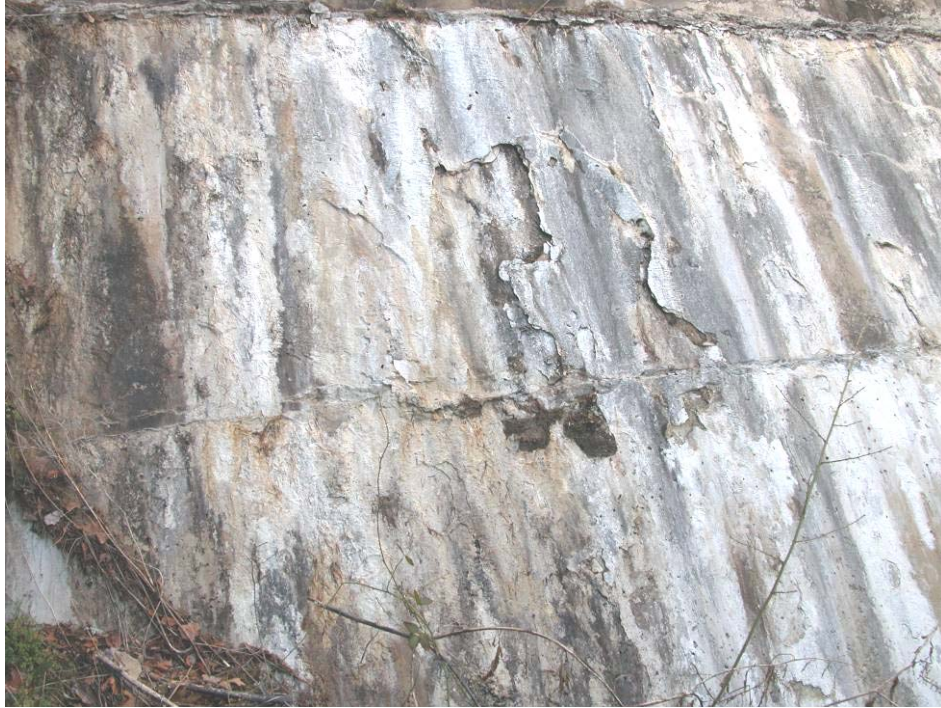
66. Afterbay Dam – View of bulging concrete and maximum efflorescence on west gravity section.
