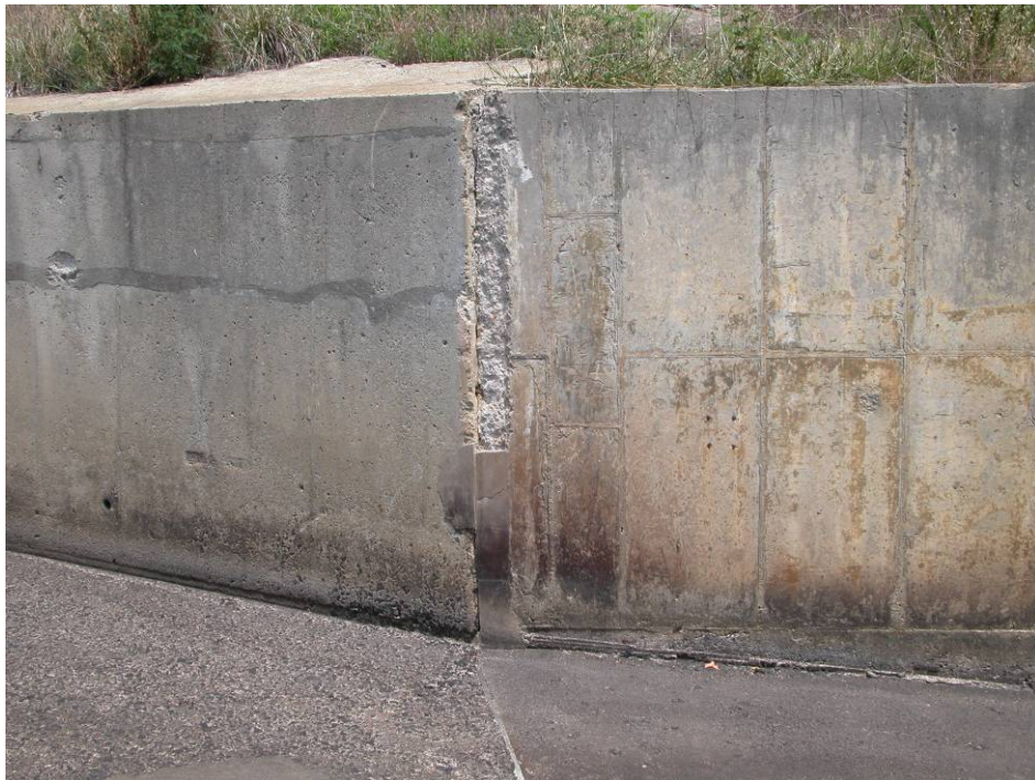
14. Main Dam – Left spillway retaining wall joint at slab J11/K12. Portion of concrete patch missing (August 5, 2008).
