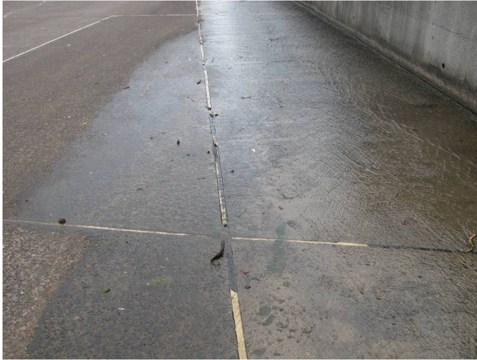
21. Main Dam – Weir flow channel caulk separated (slab F1 looking upstream - (August 5, 2008).
