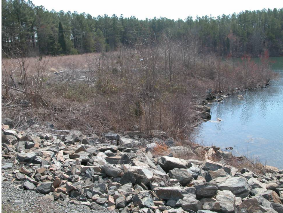
5. Main Dam – Tree growth in area of clay blanket on east upstream abutment.
