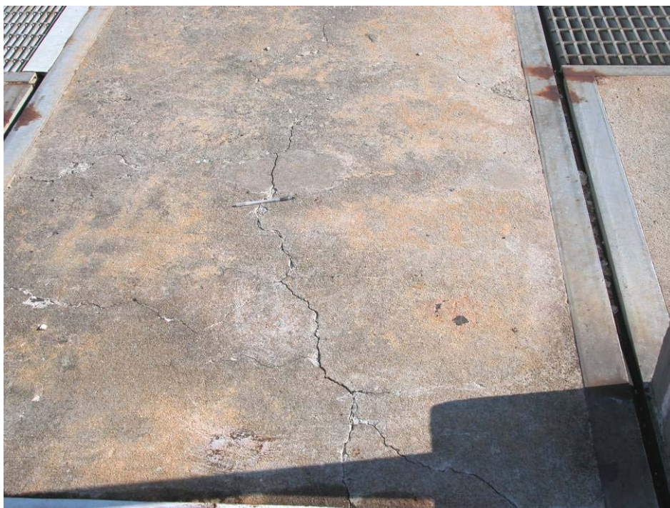
63. Afterbay Dam – View of cracking at crest of Pier 3.
