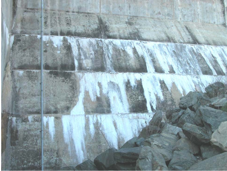
64. Afterbay Dam – View of efflorescence and minor surface scaling on east gravity section.
