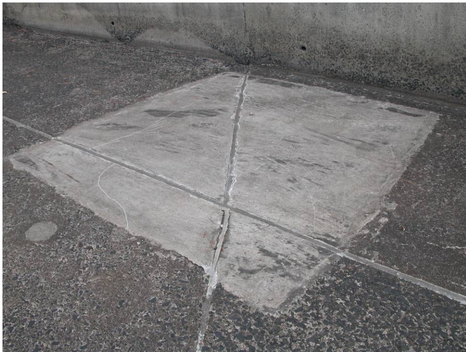
24. Main Dam – Patch over intersection G12/G13/H11/H12 has hollow sounds (August 5, 2008).
