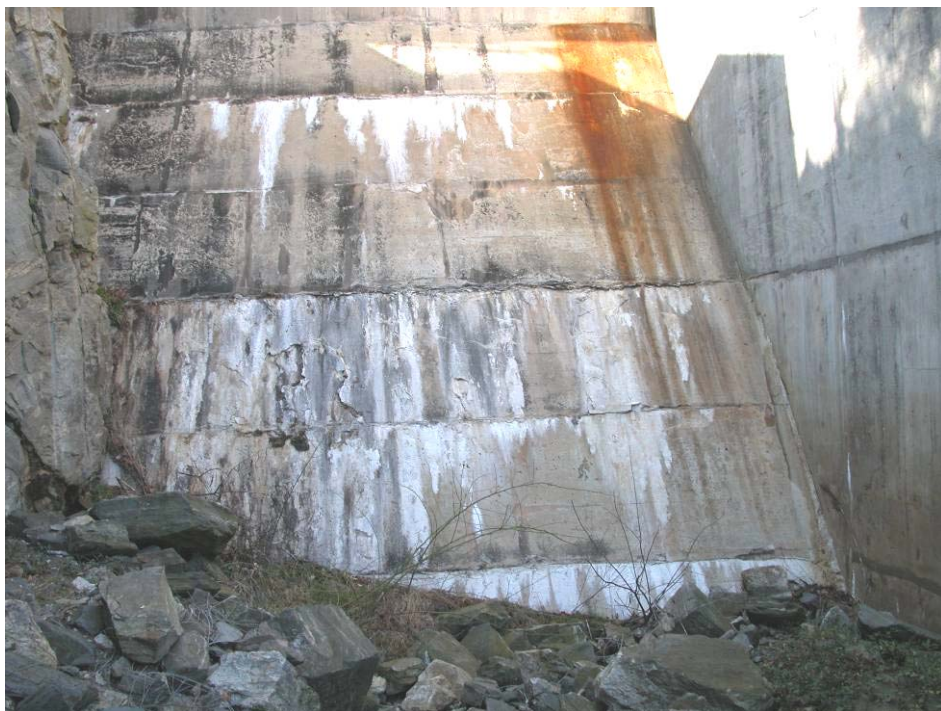
65. Afterbay Dam – View of efflorescence and minor surface scaling on west gravity section; slight dampness at junction of gravity section and Pier 5.
