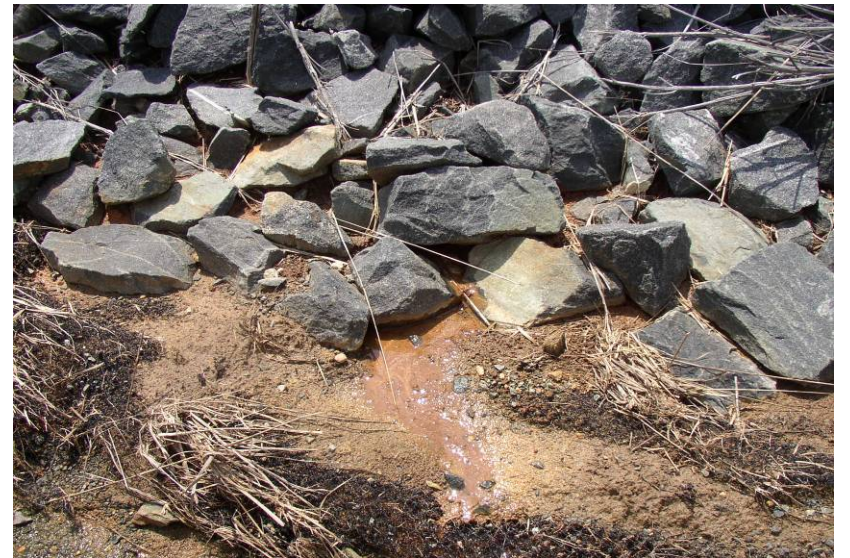
#34 Minor Local Clear Seepage Discharges from Downstream Rock Toe at South End of East Dike
