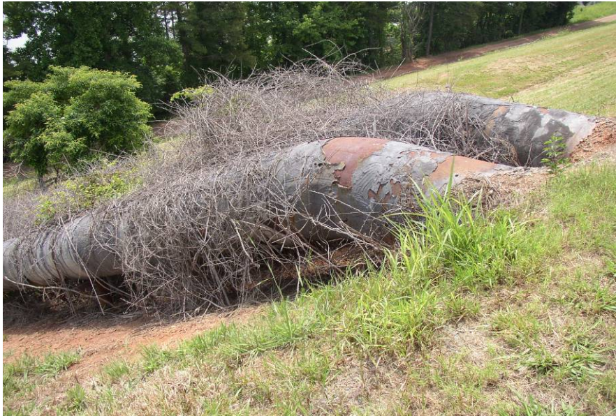
#16 Wastewater Sump Discharge Pipes @ Cell 3
