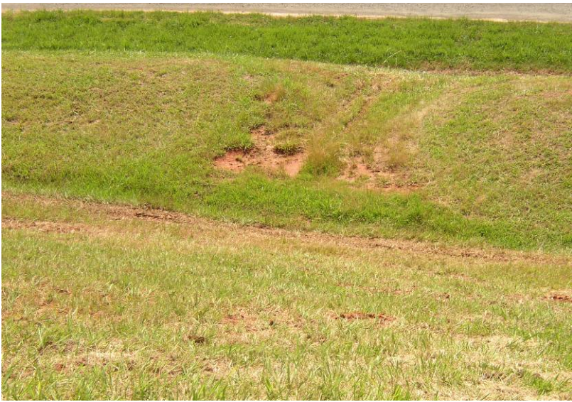
#4 Local Erosion on Top of Downstream Stability Berm – Southern Portion of East Dike
