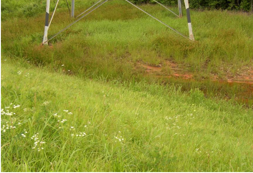
#68 Poned Water Near Downstream Toe of North Dike
