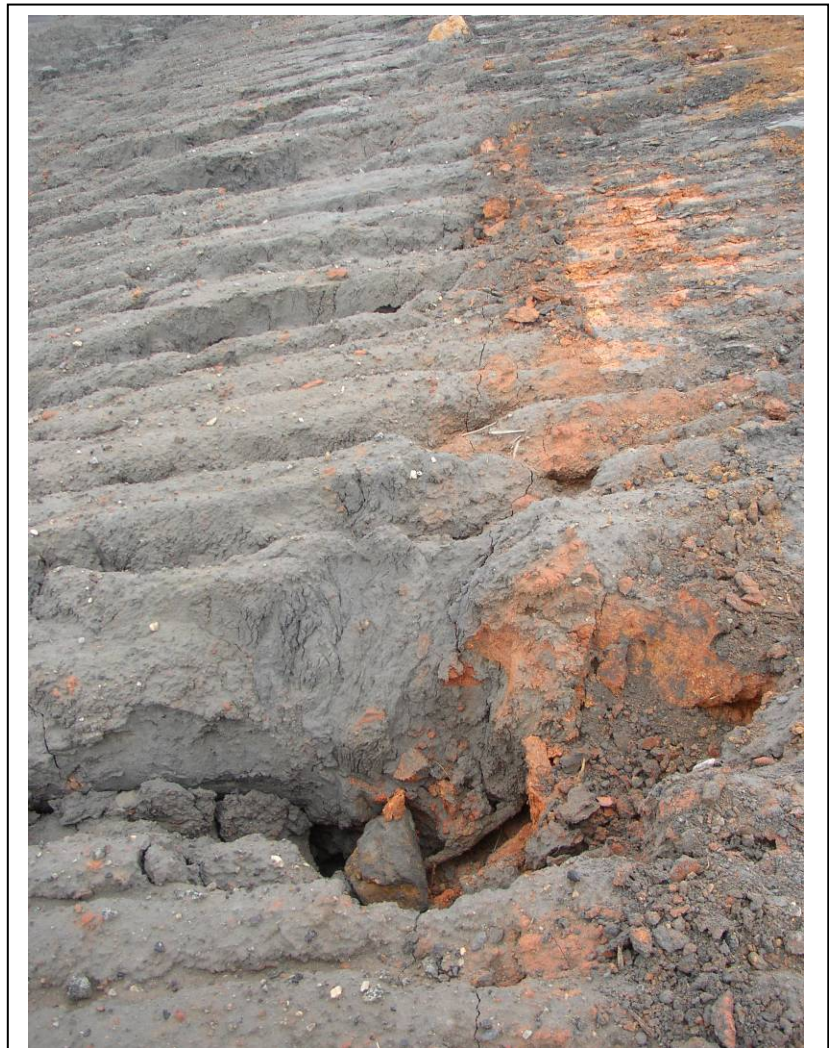
#59 Erosion in Ashfill in Upstream Excavated Slope of Cell 3
