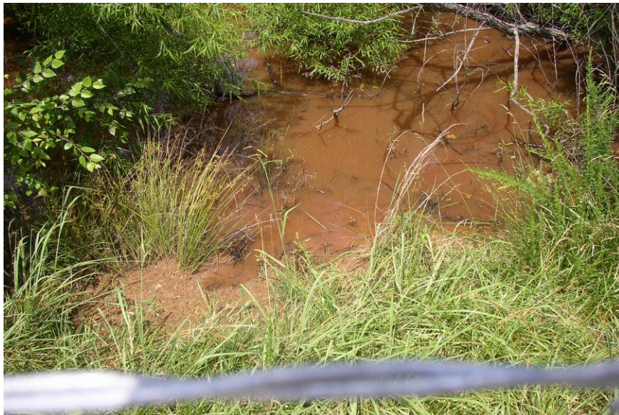
#32 Ponded Surface Water East of Downstream Toe Near Outlet
