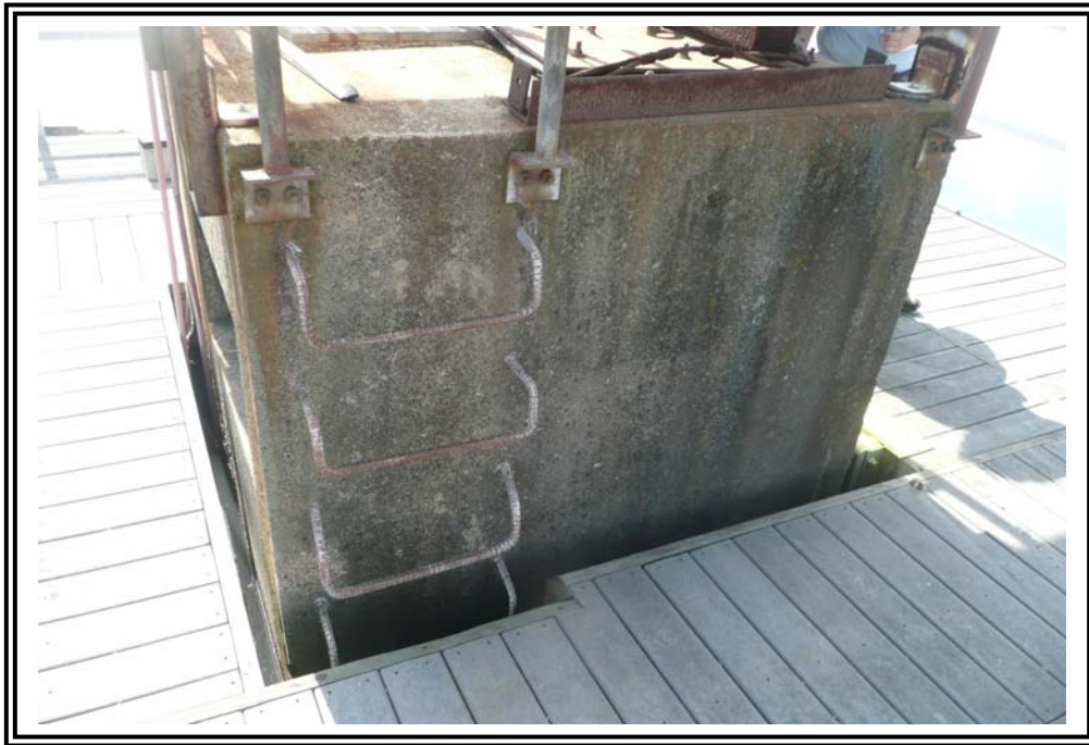
Intake tower in secondary pond.
