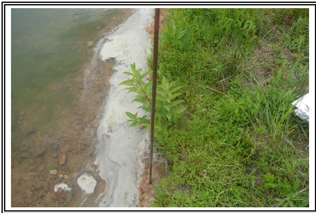
Upstream slope intermediate dike beach erosion. Floating material is composed of cenospheres.
