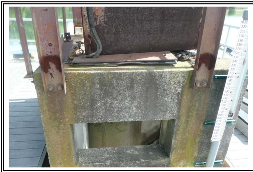
Intake tower in secondary pond.
