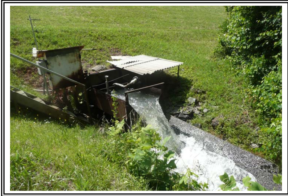
Outlet structure at toe of secondary dike, looking upstream to the south-southwest (towards secondary cell).
