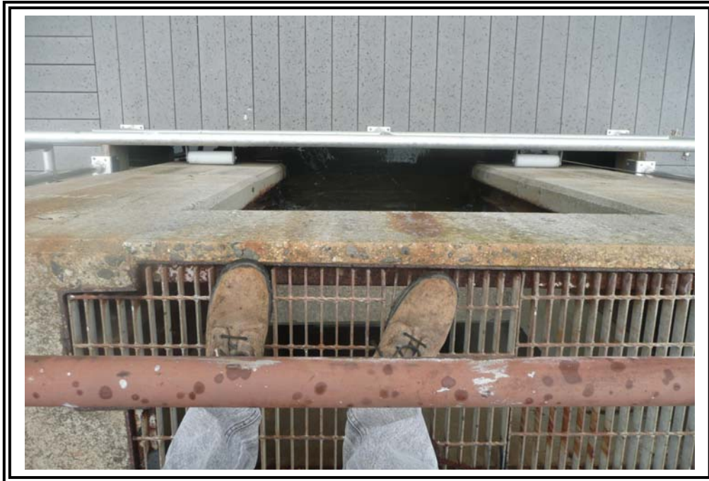
Open weir in primary cell outlet tower.
