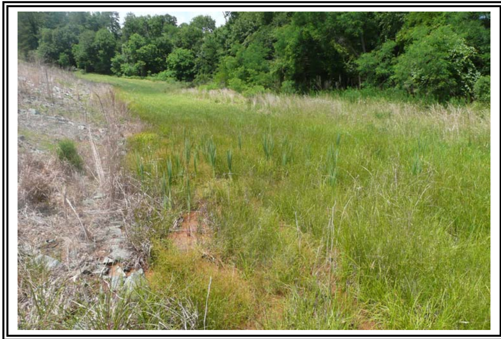
Reeds growing in area of seepage at the toe of secondary dike.
