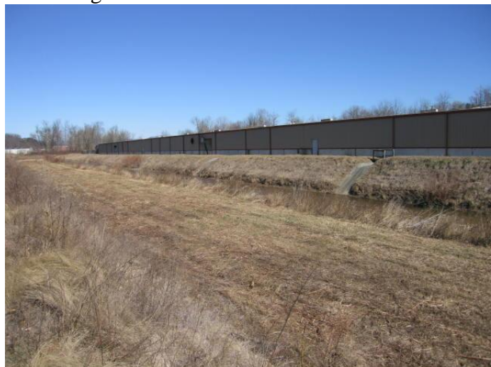
Photo 8. Breaks were common and consisted of embedded concrete lined channels. A total of 87 were counted for the entire length of engineered channel.
