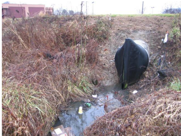
Photo 11. Check valve observed along Lovills Creek allows stormwater to discharge and prevents flood water back flow to upstream parking lot.
