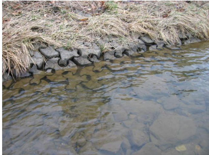
Photo 7. Interlocking concrete pavers lined stream banks to prevent erosion worked very well. None to very little stream bank erosion present along the entire length of channel.
